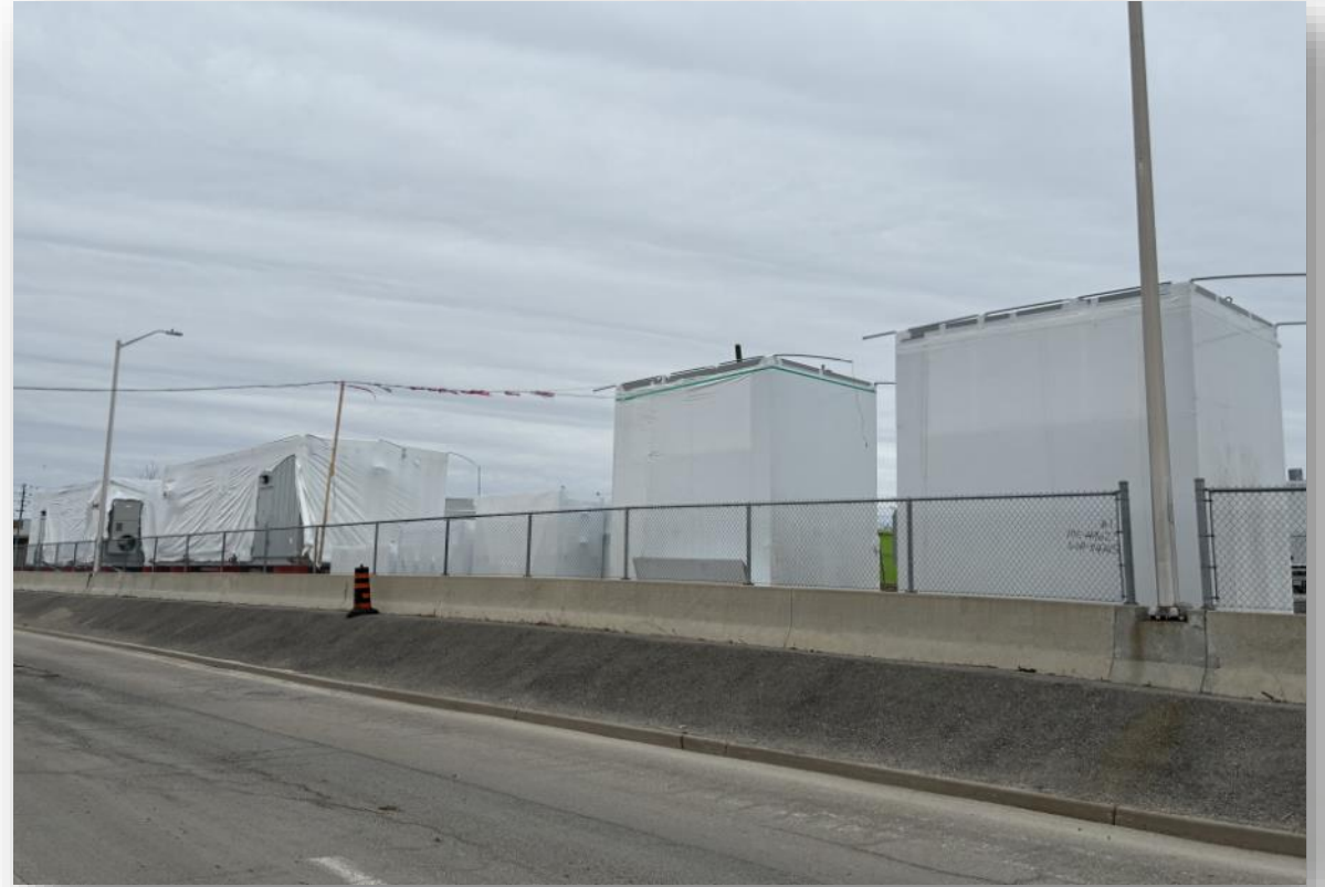
Electrical power distribution equipment
