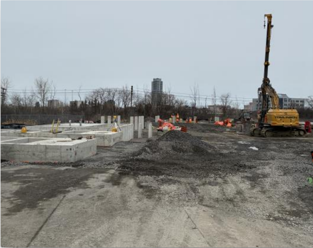
Electrical equipment foundation
