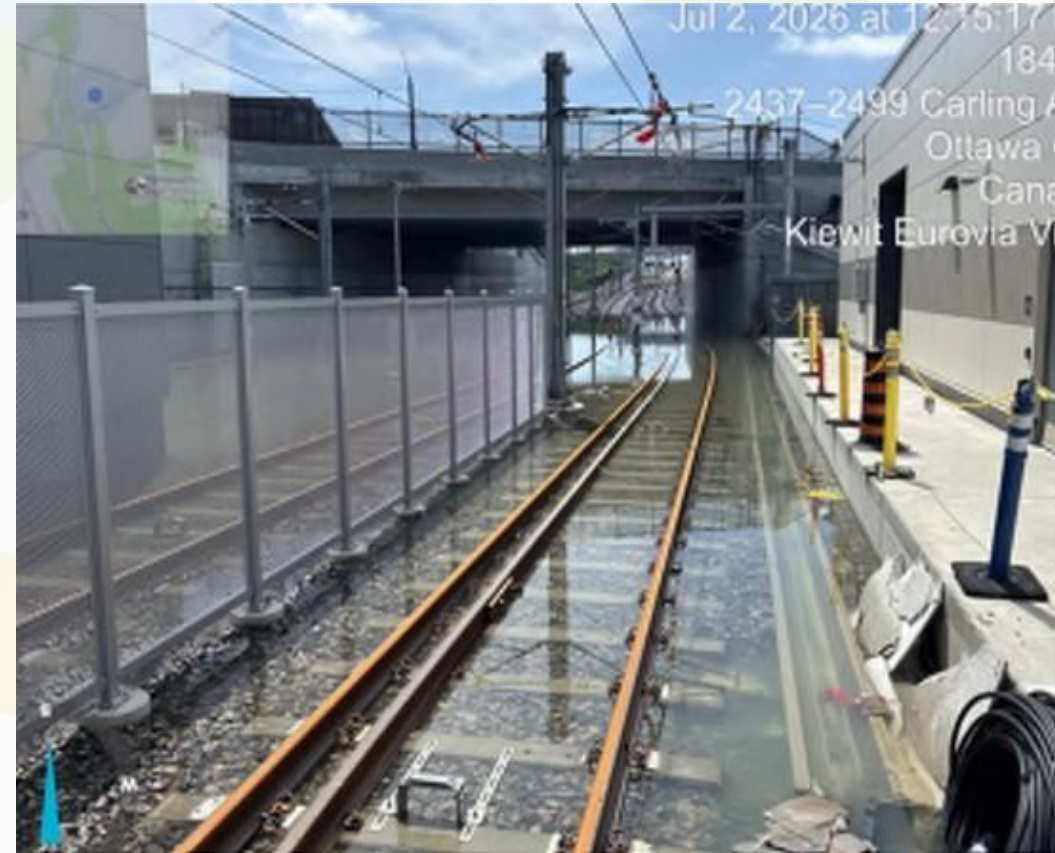
Flooding at Lincoln Fields Station
