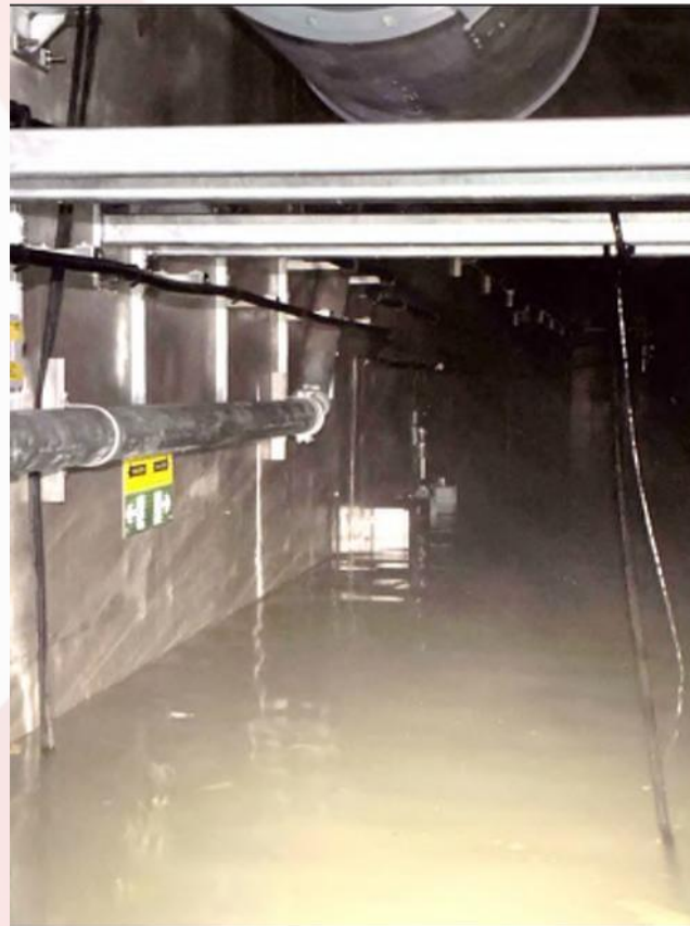
Flooding in tunnel west of New Orchard Station
